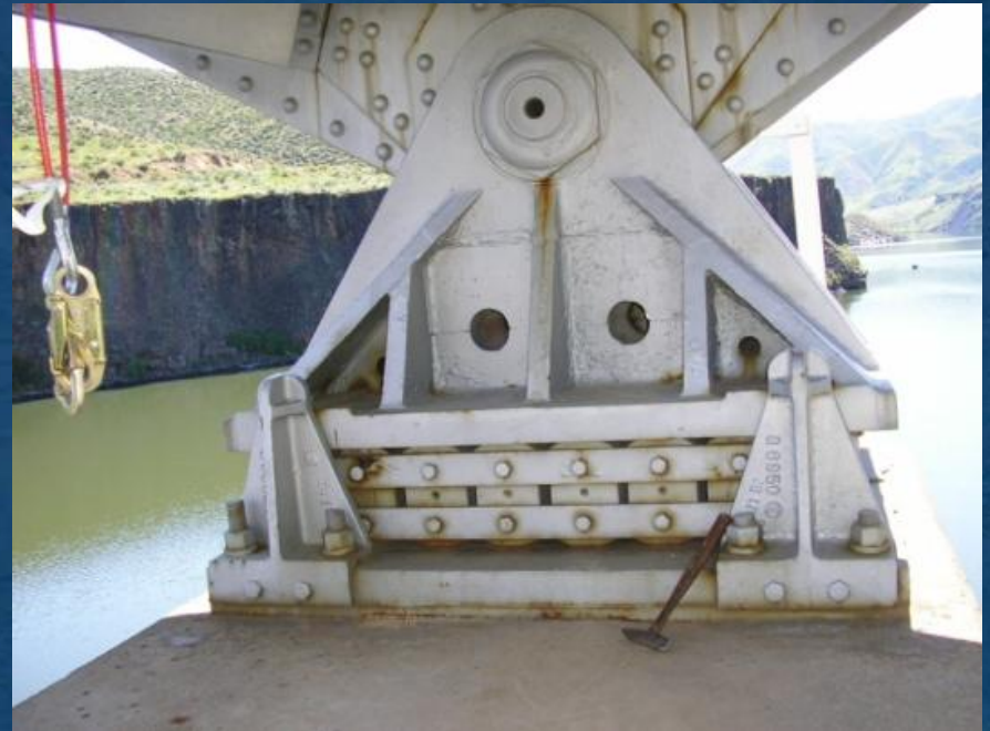
Pier 4 & 5 Expansion (Roller) Bearing
