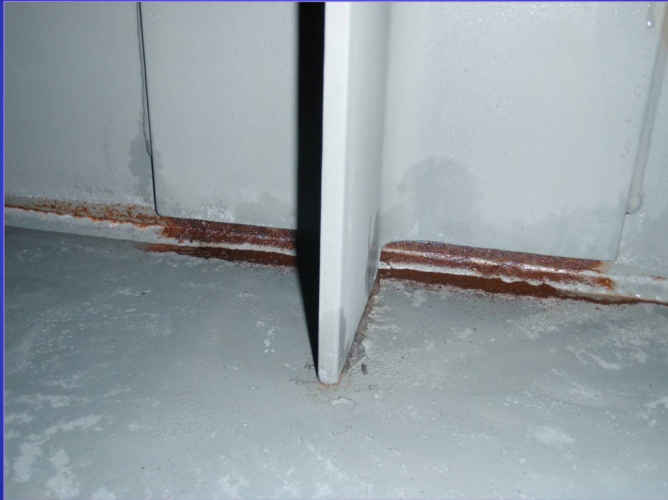
Typical Condition - Condensation
