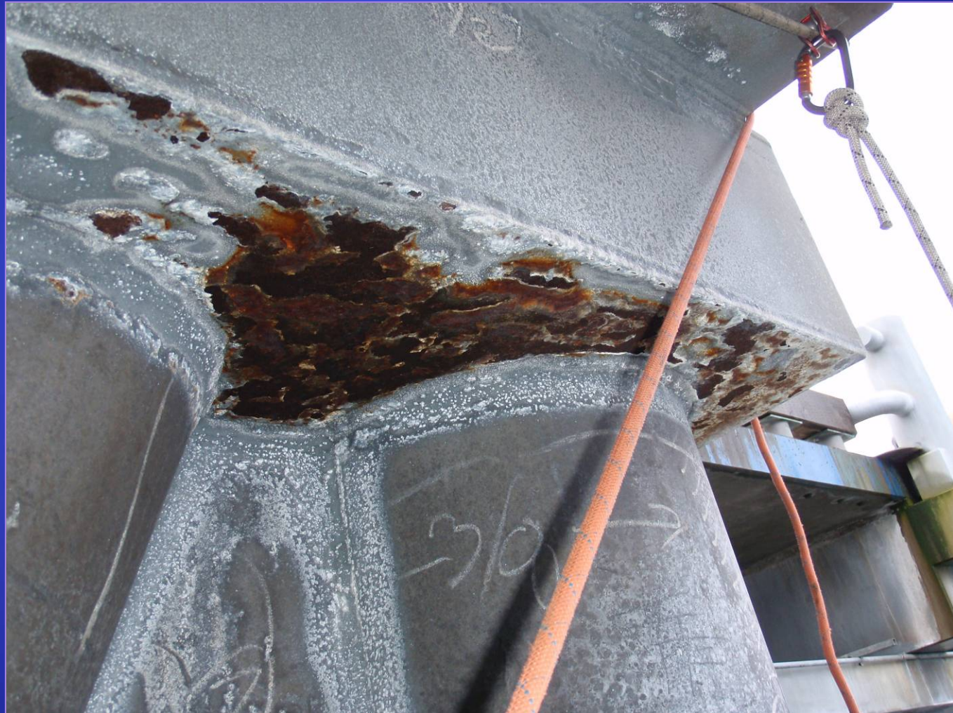
Typical Condition – Corrosion
