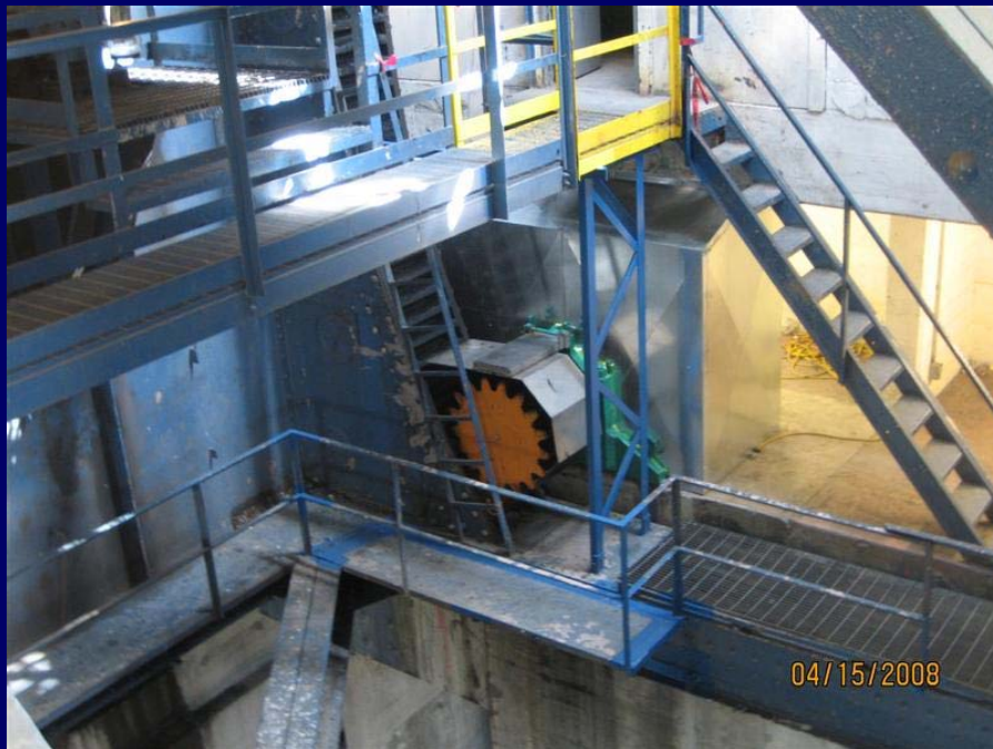
The Rack, New Pinion And Machinery Shield Viewed From Inside The Bascule Leaf
