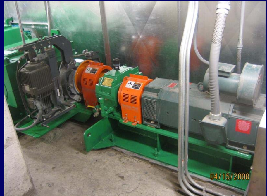
New Span Drive Motor, Primary Reducer, Motor And Machinery Brakes Viewed From The Machinery Room
