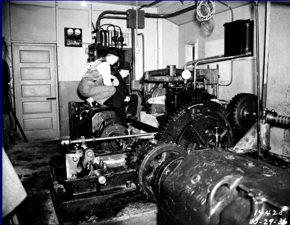
Fremont Bridge, Original Span Drive Machinery Circa 1936 Seattle Municipal Archives Photograph Collection
