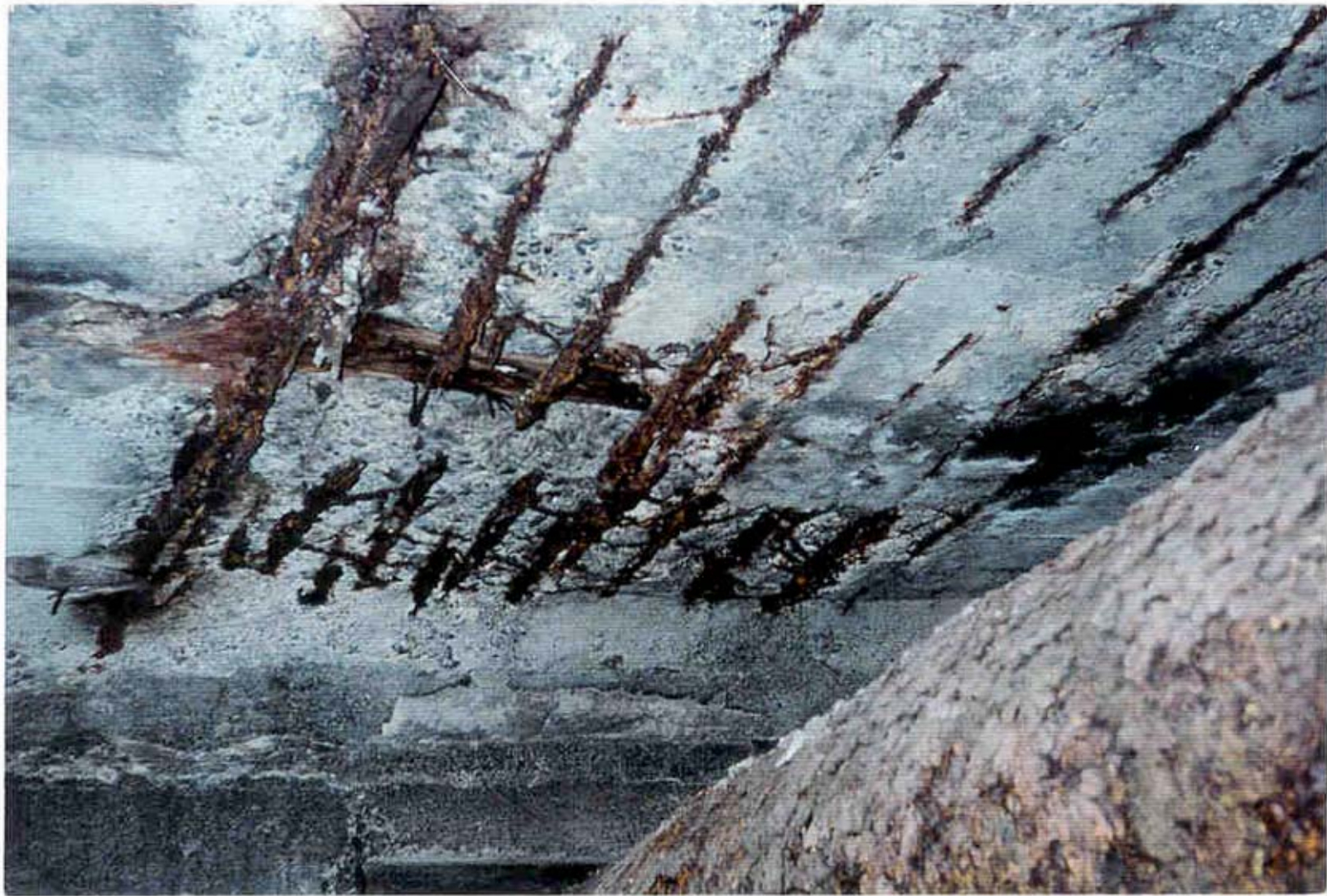
Photograph no. 3 – Looking at the underside of the deck in span 5 of the North Approach Spans. Note: Spalling concrete, exposed corroding reinforcing steel, and loss of reinforcing.
