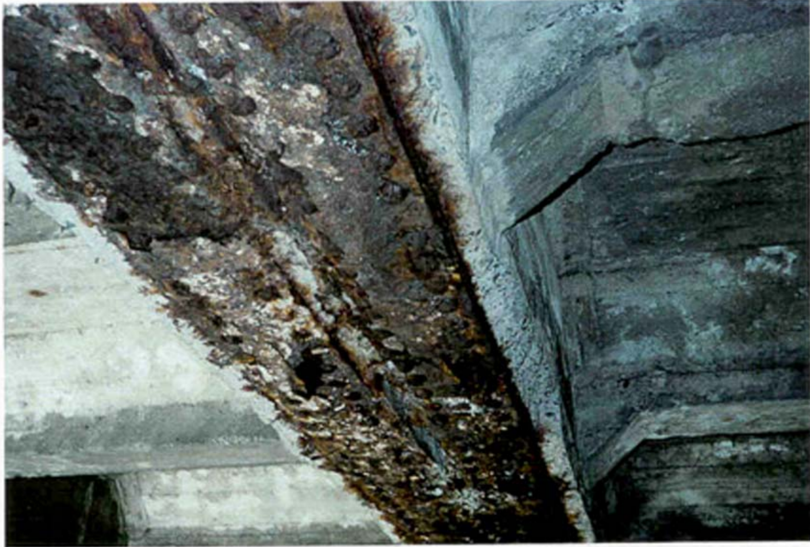
Photograph no. 25 - Looking at underside of floorbeam 14, Main Arch Span. Note: Concrete cover spalled exposing corroding steel member, rivet corrosion and loss of section.
