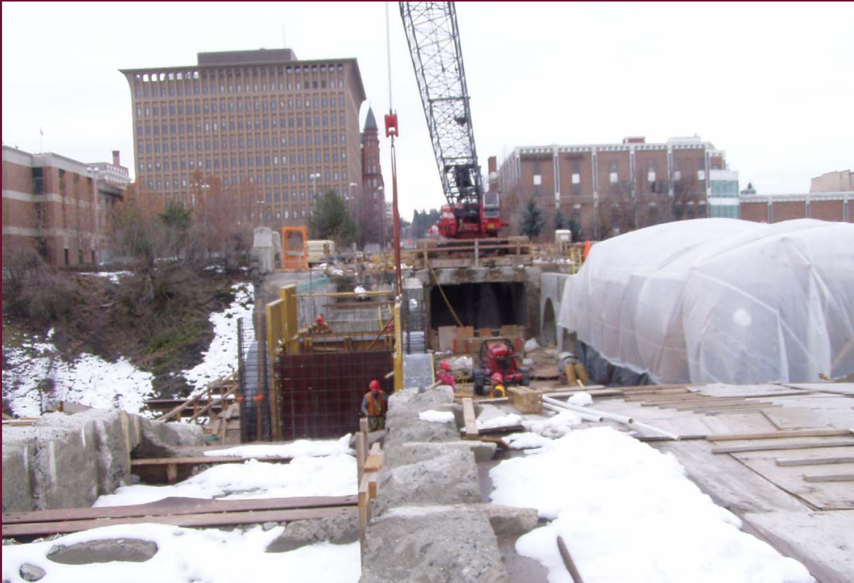
Moving Spandrel arch forms ahead from 1,2&3 to 3,&4. Notice headed pour on right.
