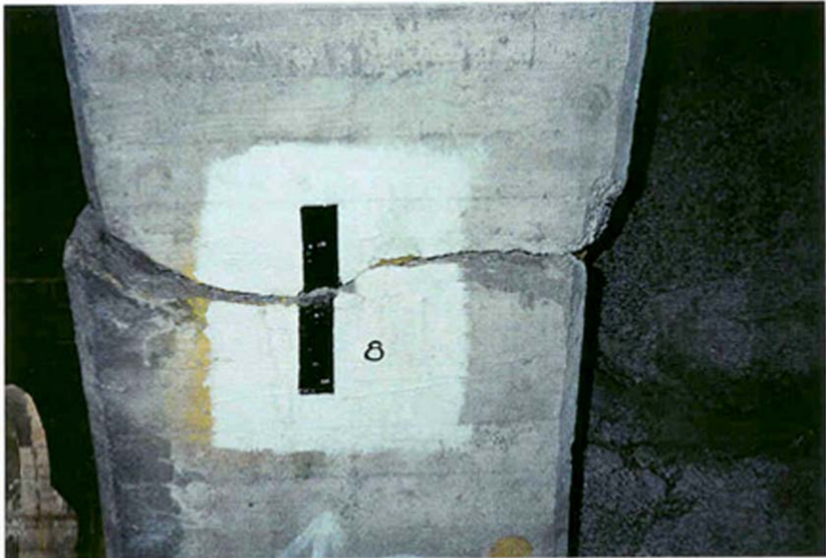
Photograph no. 60 - Looking south at pier 3 column for spandrel arch 2, North Approach Spans. Note: Severe crack width and offset.
