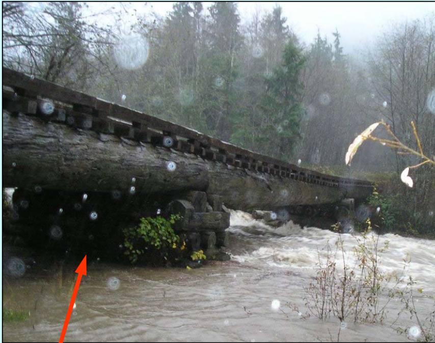
Scour Critical Piers
