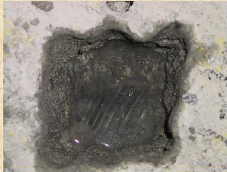
Duct w/ Water
