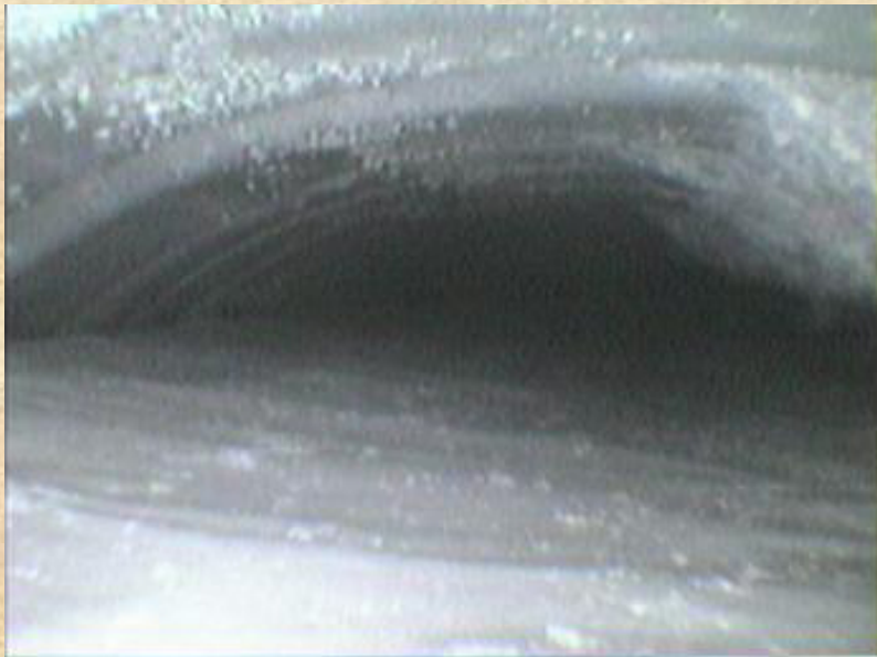
Duct w/ Void
