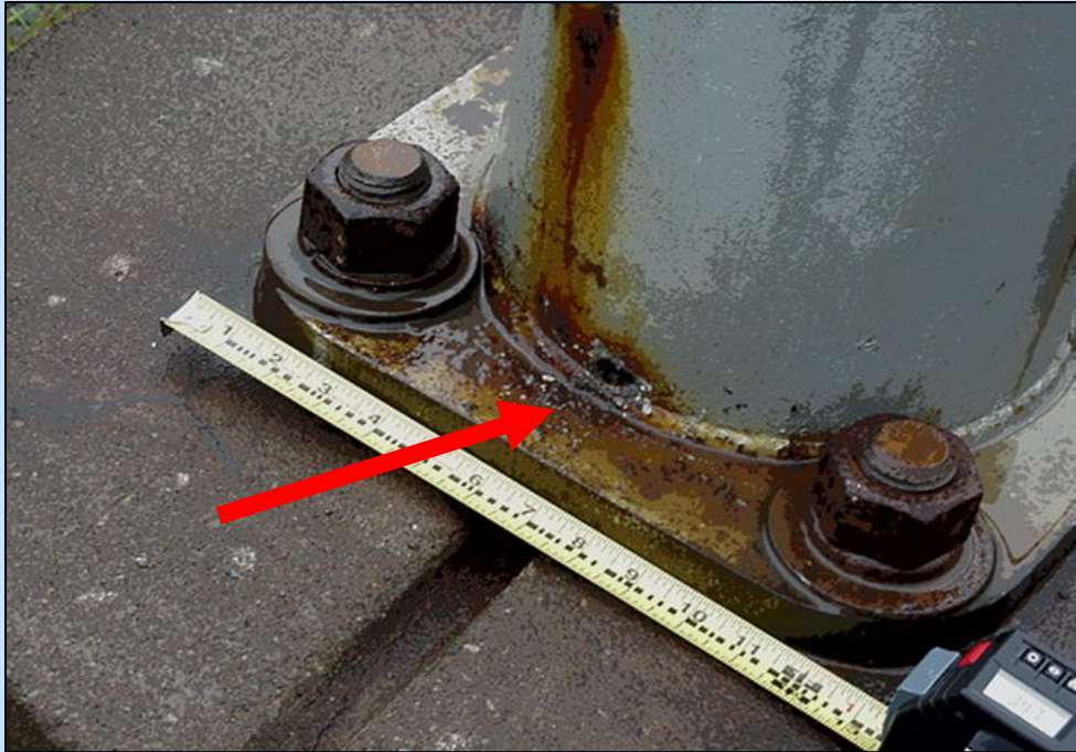
Base Plate Corrosion Note the Hole
