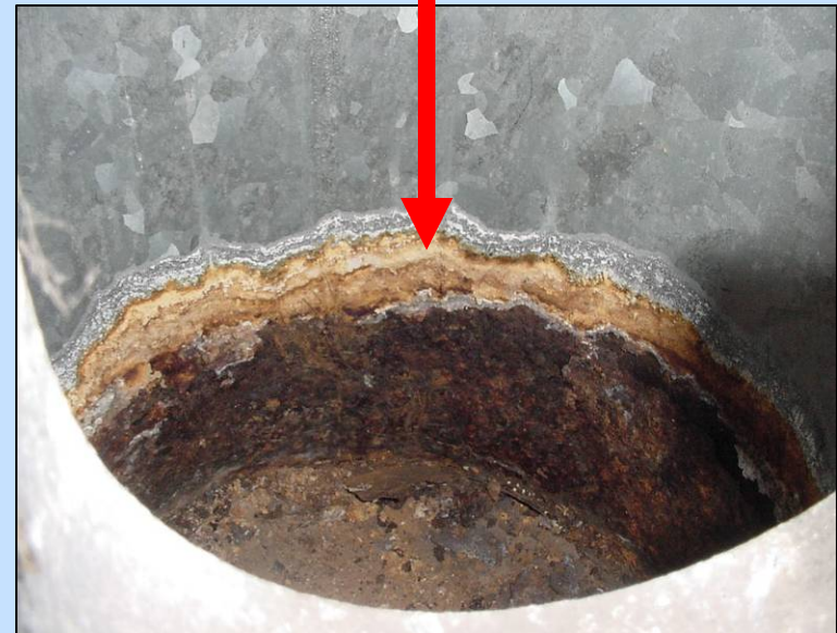
Corrosion Inside Post
