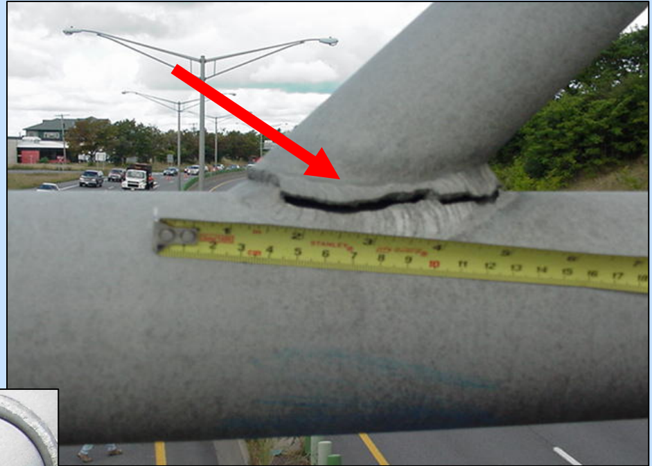
Aluminum Weld Cracks in Aluminum Truss
