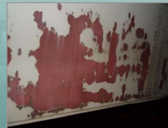
Other Inspection Findings
