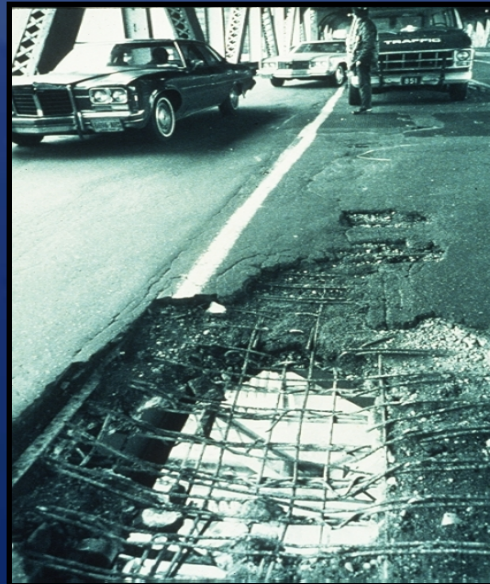
Wearing Surface Provided Little Protection
