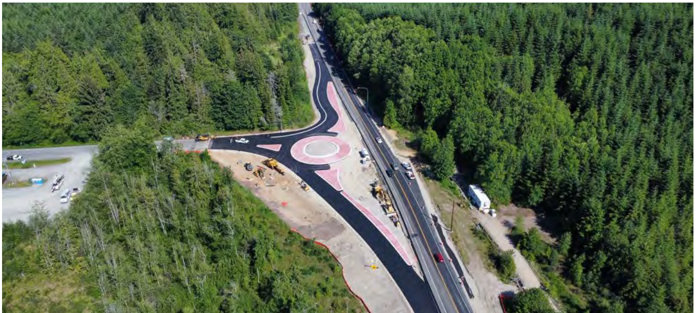
Contractor crews make progress on the State Route 19/State Route 104 roundabout in Jefferson County in June 2024.
