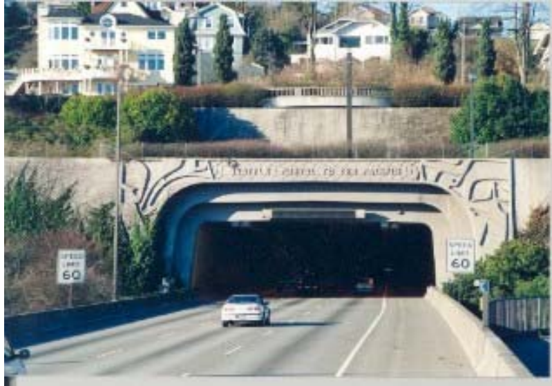
Figure 910.5 Tunnel portals can be an ideal location for a statement of community identity
