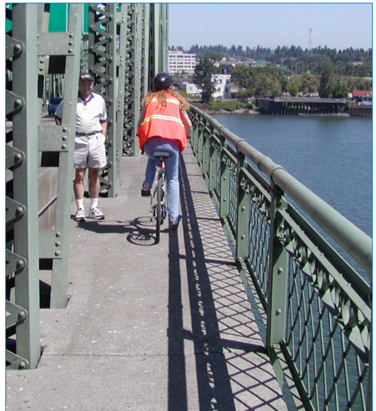
Today's Interstate Bridge paths are too narrow for pedestrians and bicyclists to safely pass each other.
