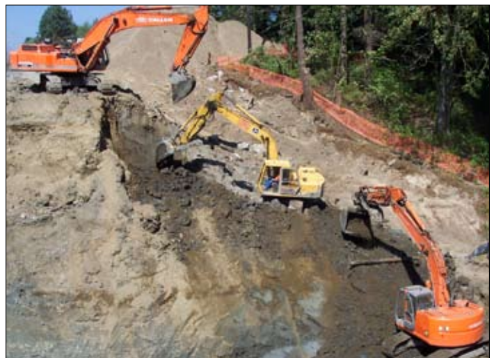
King sized bucket brigade: Crews worked in tight spaces and on steep slopes to conserve space and limit adverse effects to the surrounding area.
