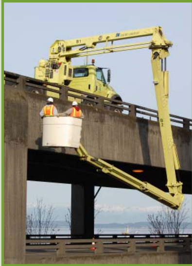
The viaduct is vulnerable to earthquakes and continues to show signs of age and deterioration. It must be replaced.
