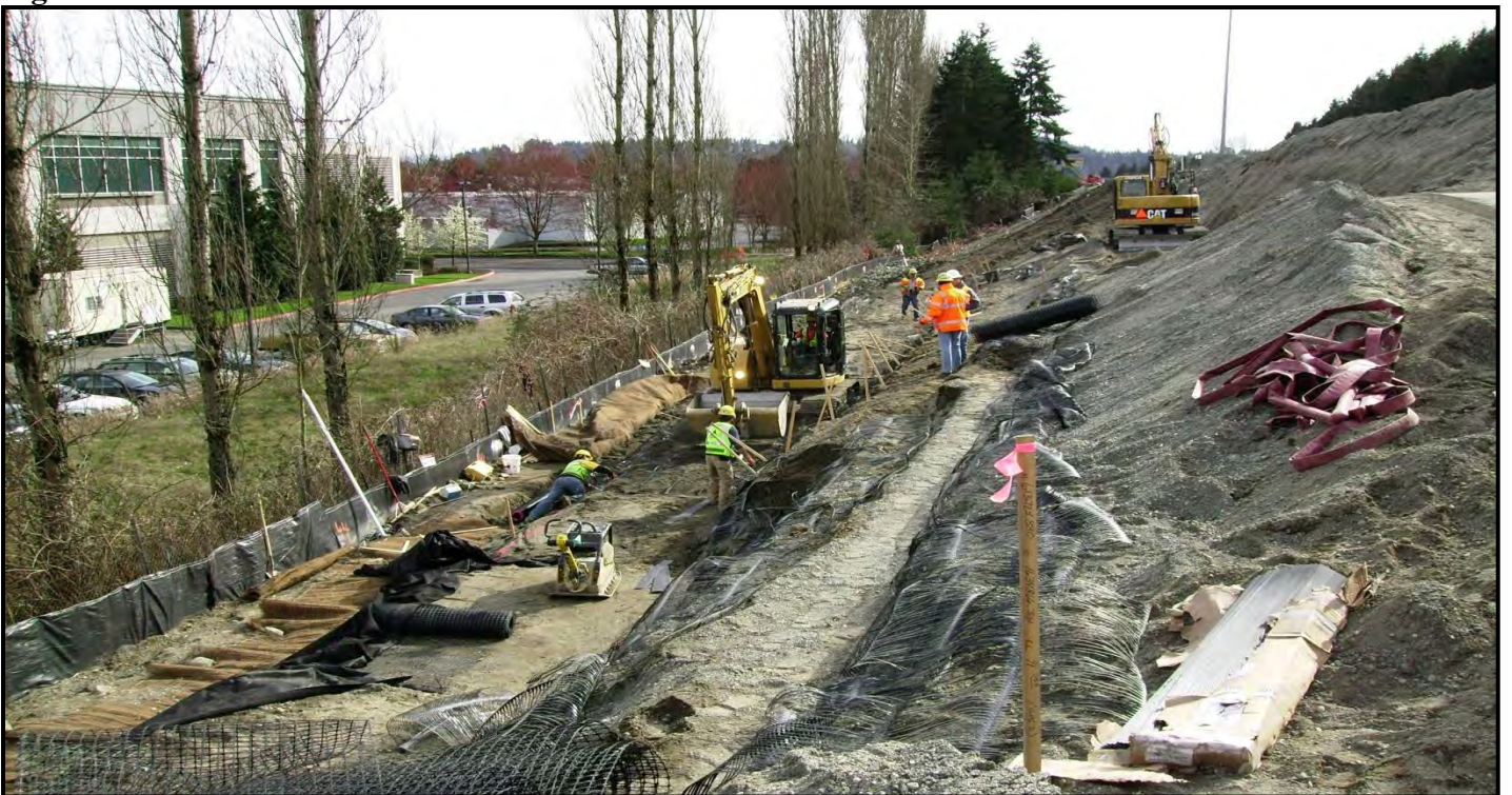
Kiewit crews in the beginning stages of construction of the 1.2:1 reinforced slope. Source: Kiewit I-405 Bothell Project photo log.
