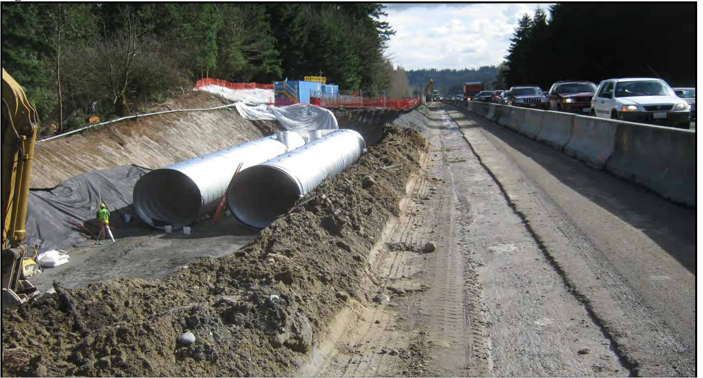
Kiewit crews begin installation of two underground stormwater detention vaults. Source: Kiewit I-405 Bothell Project photo log.
