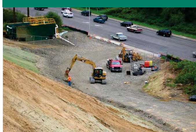
Figure 21. Quarry spalls filtration system.
