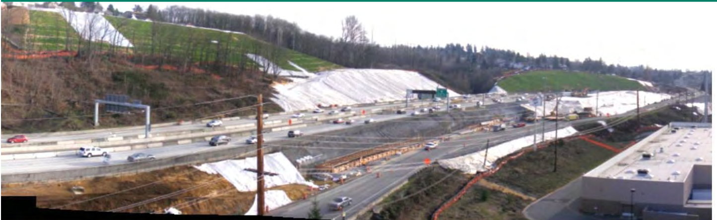
Figure 14. Cut and fill slopes were green and stable in time for the rainy season.
