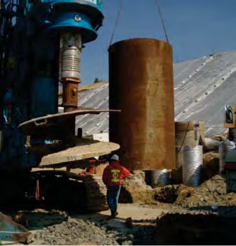
Figure 16. Diversion well casing, cut-off wall, and observation casing at abandoned mine shaft.
