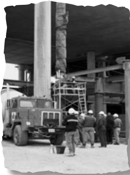
SCC delivery in Toronto for bottom-up pumping of 101-foot-high steel-form, steel-reinforced columns that were only 28 inches in diameter.
