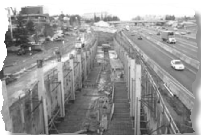
Photo 6 – A mere 10 weeks later, the bottom of the trench for the new collector-distributor lies approximately 20 feet below freeway level. Columns and footings are being placed in the trench for the new southbound off-ramp.
