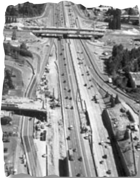
Photo 2 – Again looking north up I-405, in July 2003. In the foreground is the construction area for the new NE 4th Street bridge. On the west (left) side of the freeway, the southbound on- and off-ramps will be rebuilt.
