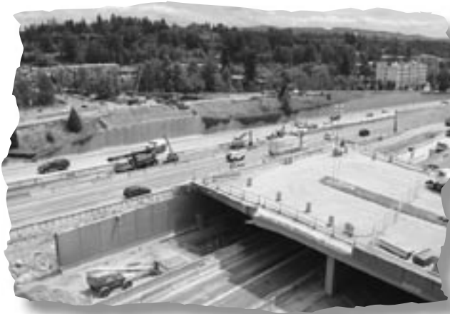
Photo 3 – The NE 4th Street bridge was demolished in June 2003. This shot was taken on July 15, looking southeast.
