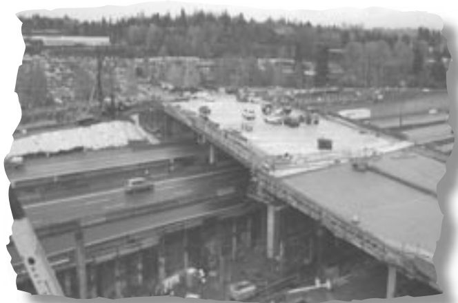
Photo 4 – Just 18 weeks after the previous shot (again looking southeast), the new bridge is in place and nearly ready to open.
