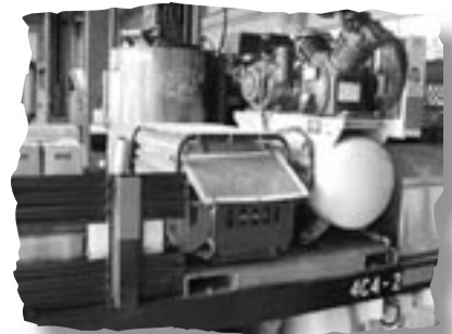
Generator, air compressor, and propane tank.
