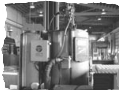
Control panel and adhesive tank.
