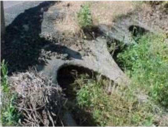
1 Culvert crossing with cleaning and flooding problems MP 359.2
