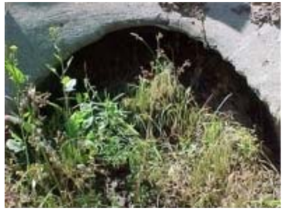
2 Culvert with annual cleaning problems MP 359.2
