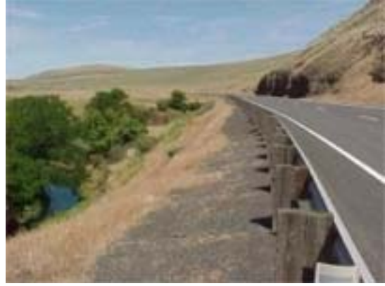
5 Unstable slope MP 383.2
