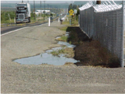
1 Improve drainage near irrigation station (MP 1.08)
