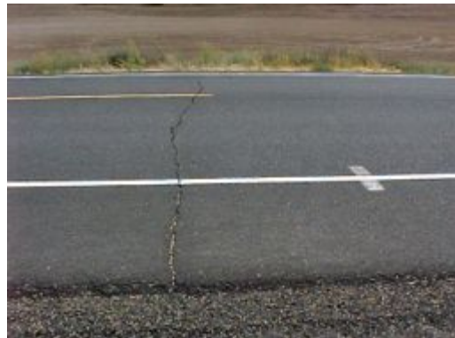
4 Cracking caused by culvert (MP 43.0)
