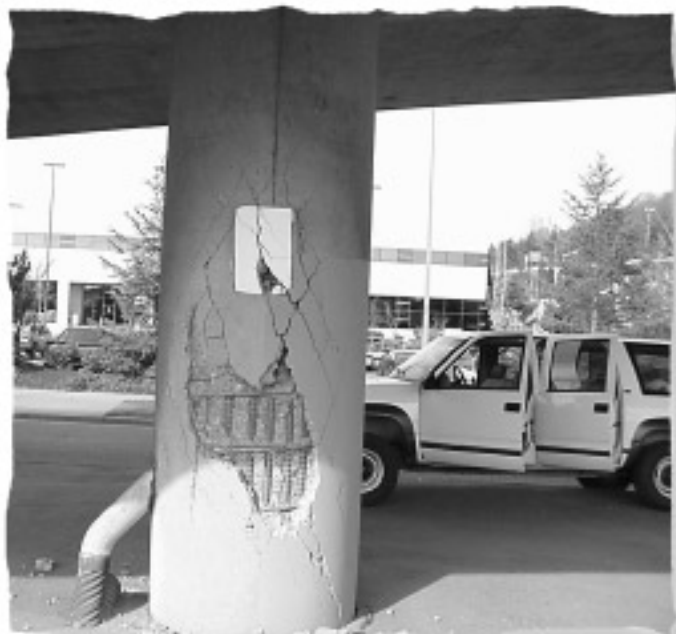
Column damage to the WSDOT's Beacon Holgate Bridge on I-90 in Seattle.
