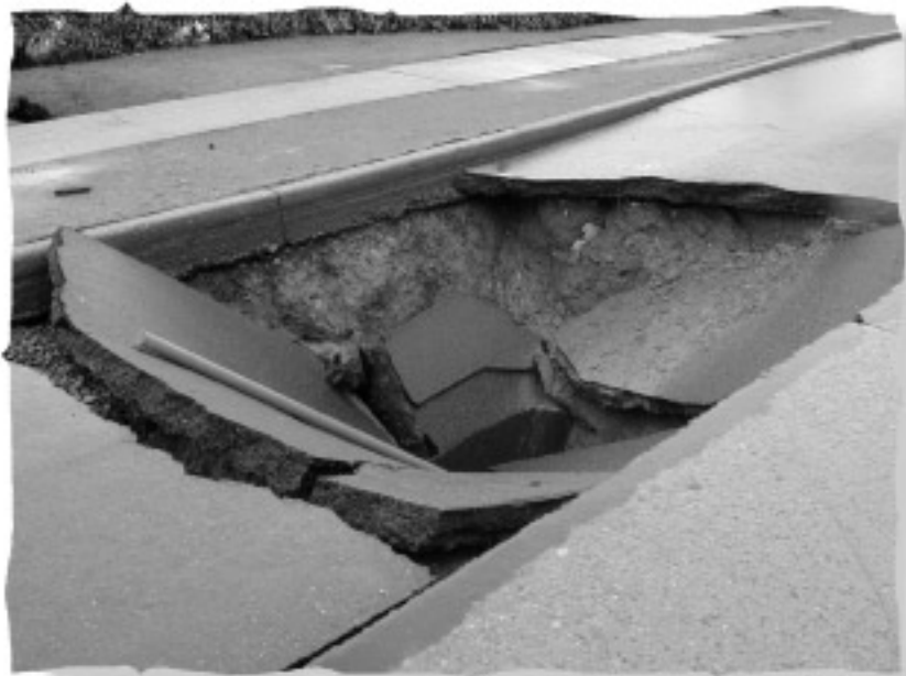
One of many sink holes along Deschutes Parkway in Olympia. (Photo by Roger Chappell)
