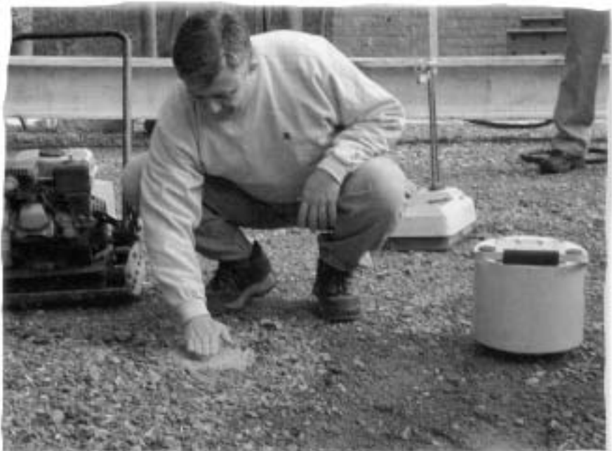
Melvin Main, who helped develop the device on the right known as the SSG, prepares the ground with a thin layer of sand to perform a soil stiffness test.
