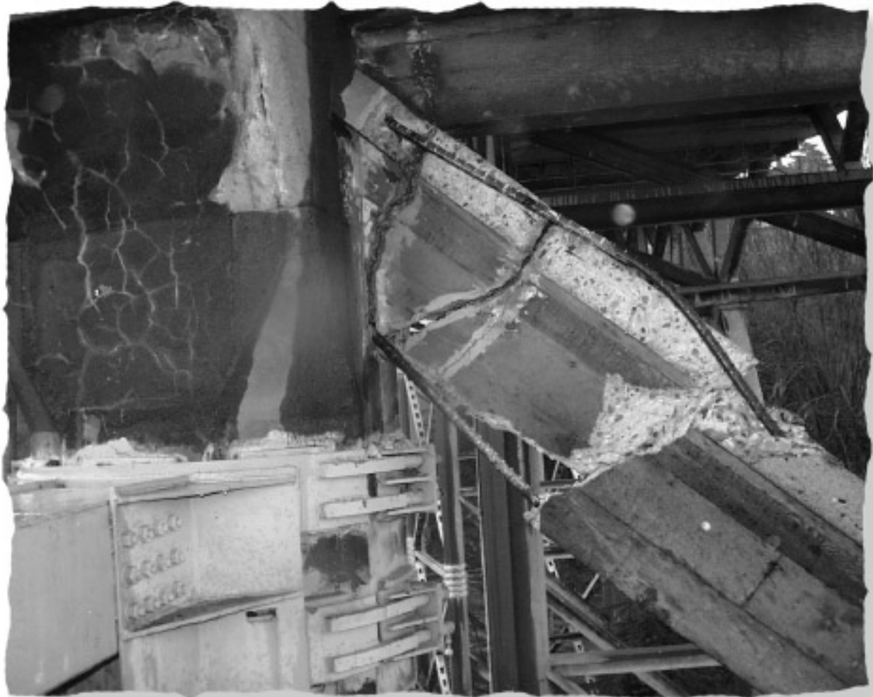
(Above) Typical damage on the City of Seattle's Magnolia Bridge. (Photo courtesy of Richard Miller, City of Seattle)
