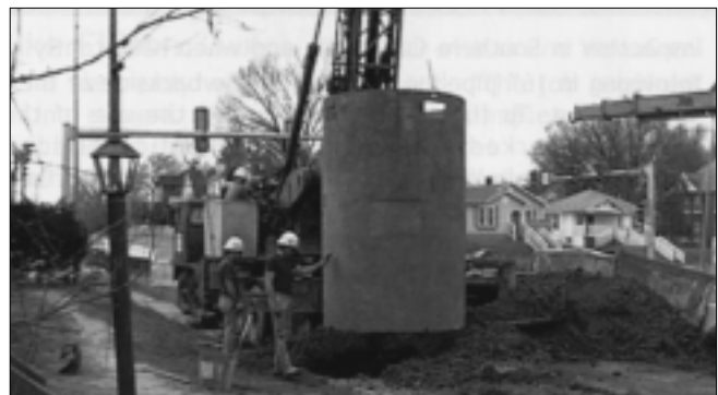
▲ An 8-ft steel can is inserted into the auger-excavated shaft. When finished, flowable fill is poured and the can is pulled from the shaft.
