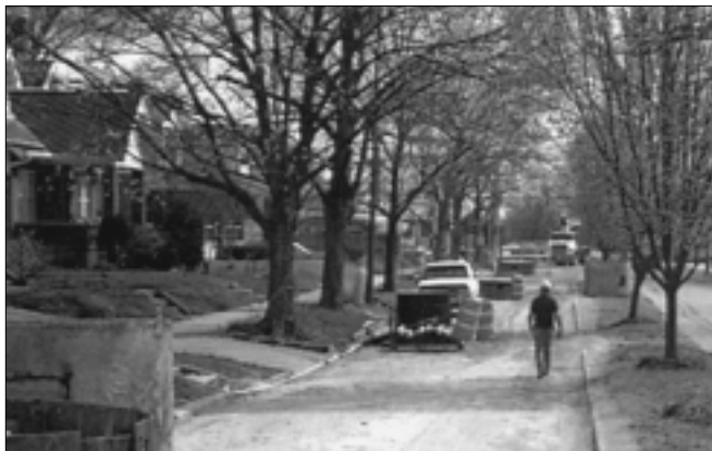
▲ The small pilot tube microtunneling system enabled Cape Girardeau to install more than 40,000 lin. ft. with disturbance of only one tree.
