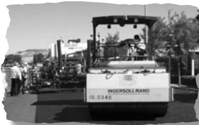
Photo 9 – Compaction should be started immediately after placement and be completed before the mix reaches 195°F.
