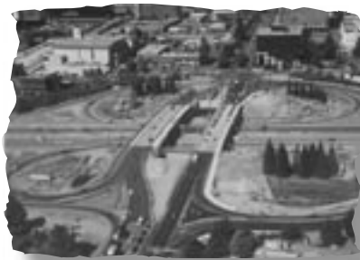
Summer 2003. Both halves of the new bridge with the gap in between, where the old south half was demolished. The new south half (on the left) will be rolled across the gap.
