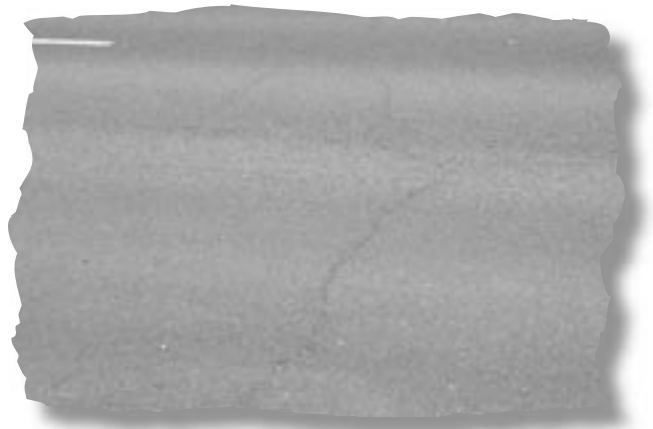
Photo 12 – Transverse crack reflecting through the NovaChip® overlay.
