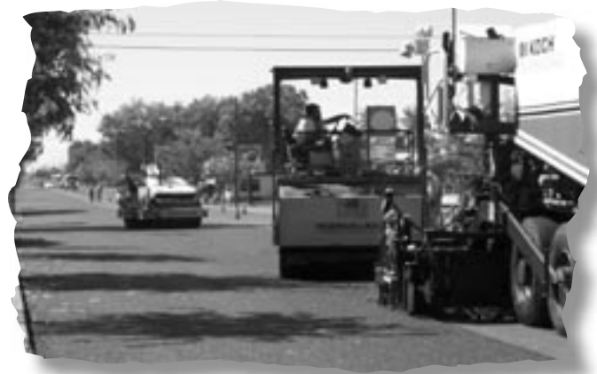
Photo 10 – Compaction was obtained by the use of two static double drum rollers.
