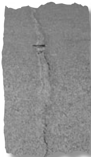
Photo 3 – Cracks of this severity (greater than ¼ inch) should be sealed or repaired prior to the NovaChip® overlay.
