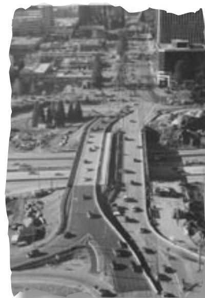
Late 2002/early 2003. The new south half of the bridge is on the left; the old south half is on the right. The old north half has been demolished and construction is underway on the new north half.
