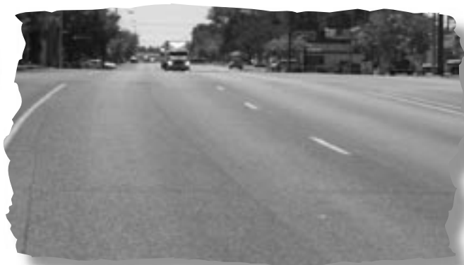
Photo 2 – A portion of SR 17 through Soap Lake in eastern Washington prior to the application of NovaChip®.
