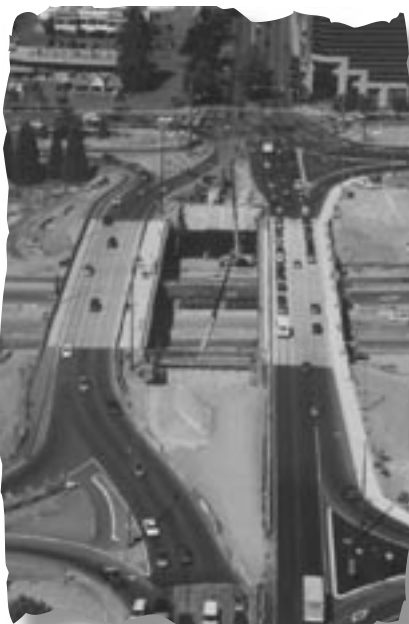
Eastbound traffic (on the left) jogs over to the south half of the bridge; after the south half is relocated, traffic will flow smoothly straight through.
