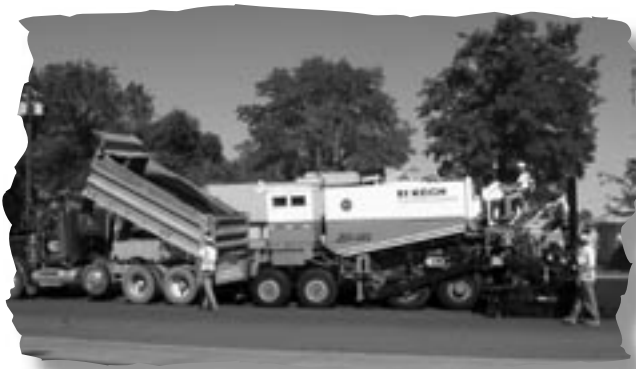
Photo 7 – The “Novapaver” is capable of placing the NovaChip® and the Novabond® membrane in a single pass.
