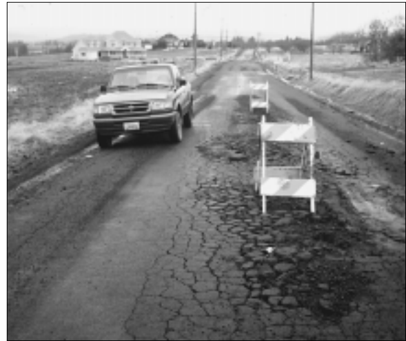
▲ Original road condition
