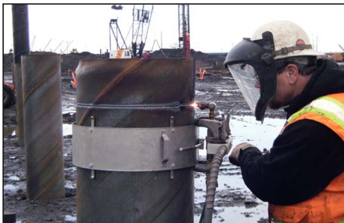
A steel worker uses precision instruments to create a clean cut on a recently driven pile.
