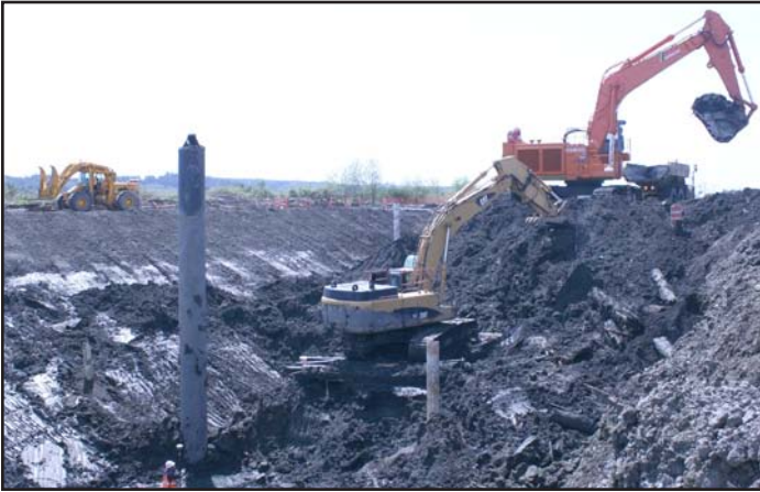
Crews use heavy machinery to excavate the casting basin one scoop at a time.
