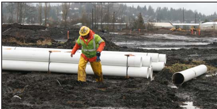
During the wet winter in Aberdeen, crews worked to dewater the site by constructing wells using PVC pipe.
