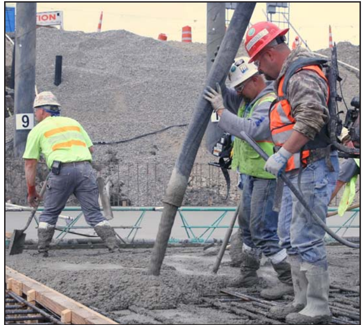
Concrete workers place 660 cubic yards of concrete to form the first base slab of the casting basin.
