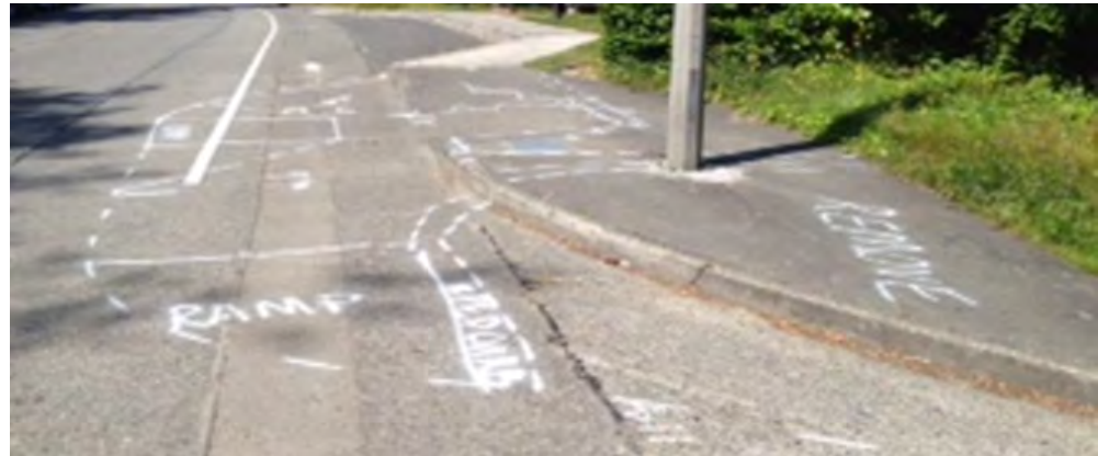
A curb and sidewalk that have been marked with white paint to indicate where a new curb extension and curb ramp will be installed.
