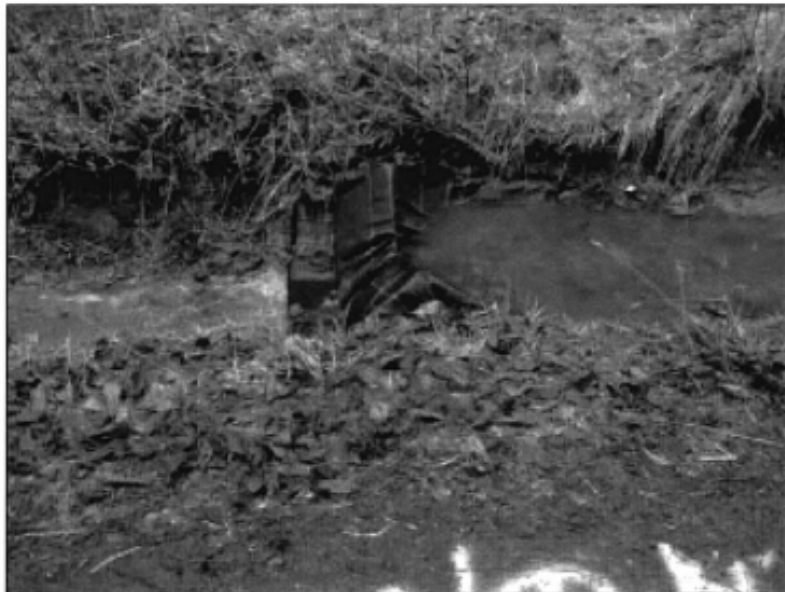
A triangular silt dike in place with accumulated sediment being retained on site, prior to cleaning
