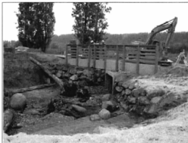
Large woody debris placed in streambed to provide fish refuge. Note use of streambed gravel, mulch, and coir fabric
