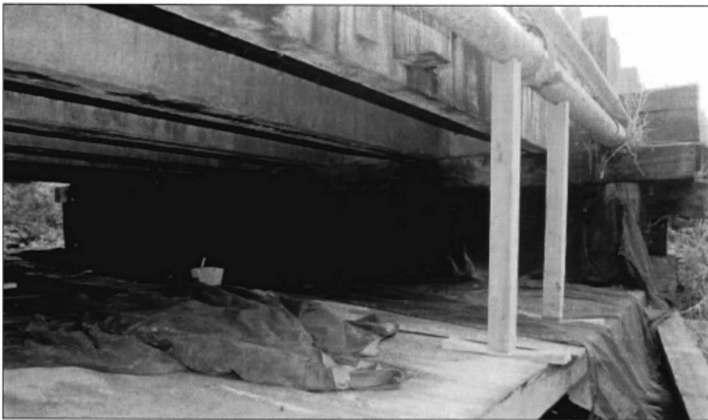
Plywood work platform providing a safe work environment and containing fallen debris from entering water during construction, maintenance, and repair activities
