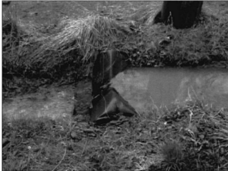
A triangular silt dike detaining water and allowing soil particles to settle
