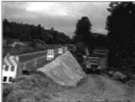
Plastic covering used as erosion protection on a slope at construction/repair area. Note additional use of mulch in area
