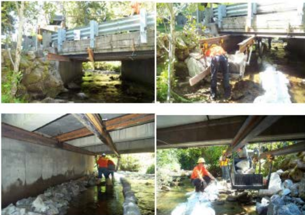
Bucket tram used to transport rip rap for a bridge scour repair.
