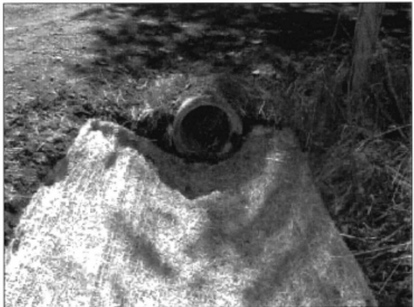
Silt mat installed in ditch to decrease erosion and allow settlement of suspended solids
