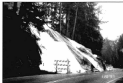
Plastic covering used as a temporary erosion control on slope at slide area after storm and before repair
