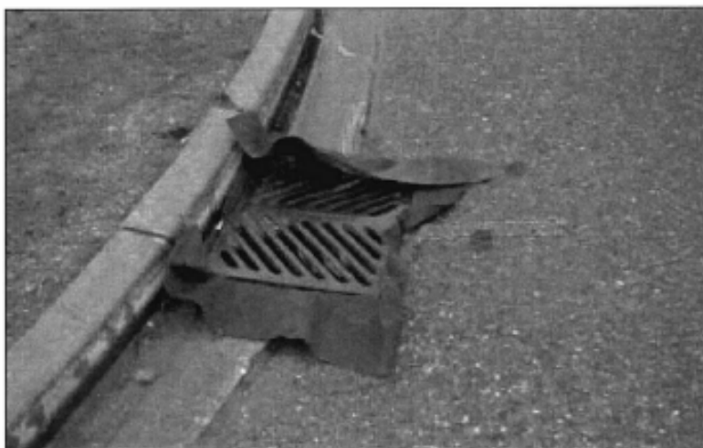
A silt sock installed in a catch basin to trap/filter waterborne soil particles
