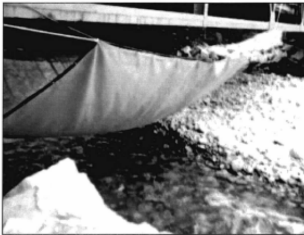
Diaper netting under bridge
