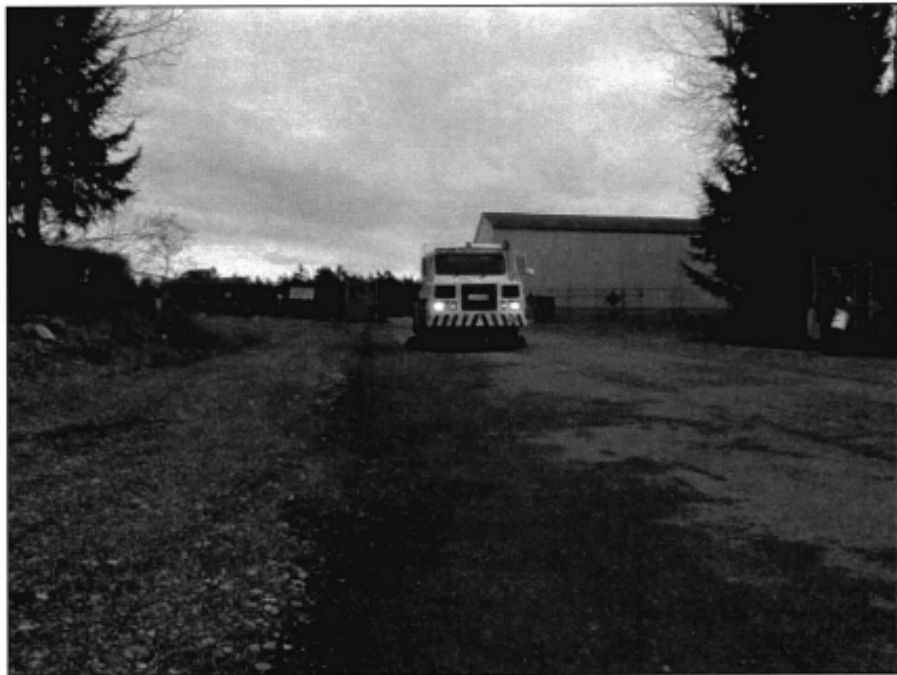
A sweeper picking up debris and soil particles on a paved access road
