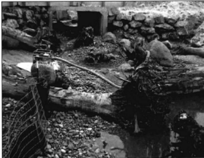
Large woody debris placed in streambed to provide salmonid refuge. Note use of streambed gravel, dewatering with pump, and mulching
