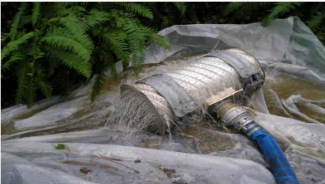
Figure 10: Outlet Energy Dissipater.
