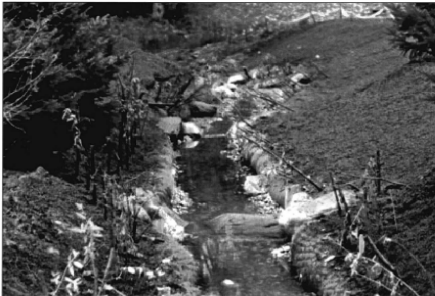
Stabilizing the stream bank by using coir logs, hydroseeding, and live staking. Streambed gravel installed to provide a natural spawning substrate
