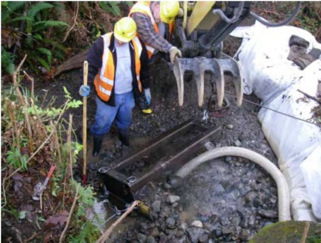
Figure 5: Pull Dozer deployed at culvert outlet. Note snatch block mounted to excavator bucket used to mount cable pulling the dozer through the culvert and the smaller cable mounted at the rear used to pull it back into the culvert.
