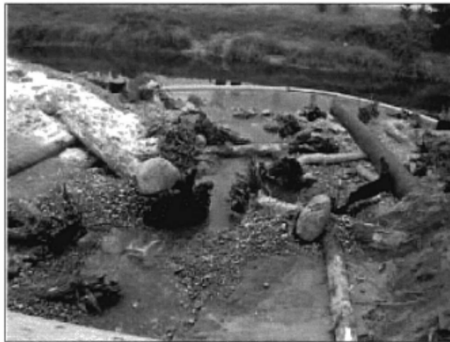
Large woody debris placed in a streambed to provide salmonid refuge. Note use of turbidity curtain , streambed gravel, silt fence, coir fabric, mulching, and stream bypass
