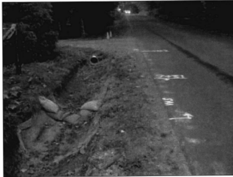
A sandbag barrier used to decrease water velocity. Note use of silt mat and hydroseeding to decrease erosion and to increase vegetation in channel
