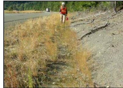
WSDOT surveyed potential jurisdictional ditches for the first phase of the project.
