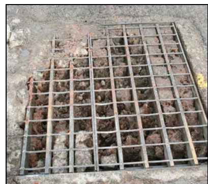
Stormwater inlets clog with snow and ice, which causes water to build up on the roadway creating unsafe conditions.
