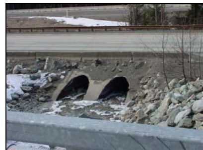
Removal of existing culverts would have long-term benefits, but would require BMPs to prevent short-term construction impacts.
