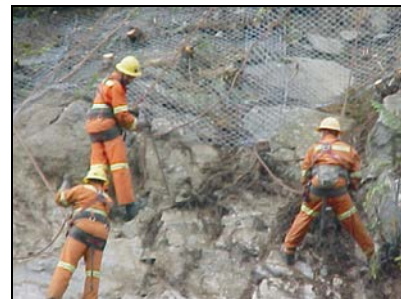
WSDOT installs rock bolts and netting to improve safety from rock fall within the project area.
