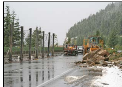
Unstable slopes cause damage to the highway, put motorists at risk, and can cause delays.
