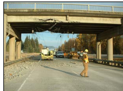
An oversized load hit the Easton Bridge outside the project limits, causing extensive damage. Similar low bridges occur at two interchanges in the project area.
