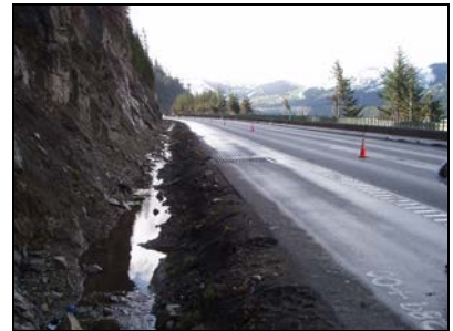
Steep slope on the uphill side of I-90.
