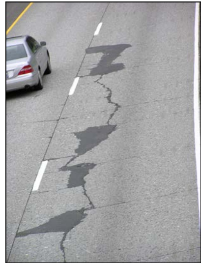
Pavement in the project area has outlived its intended lifespan and is deteriorating rapidly.
