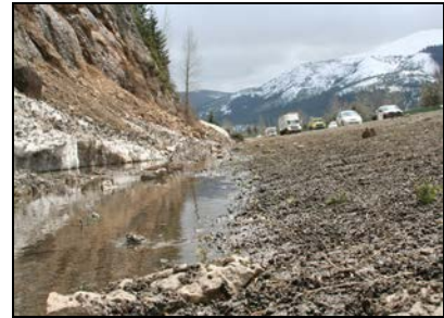
Steep constrained slopes uphill of I-90 cause snow and stormwater to accumulate in existing undersized ditches and flow to streams untreated.
