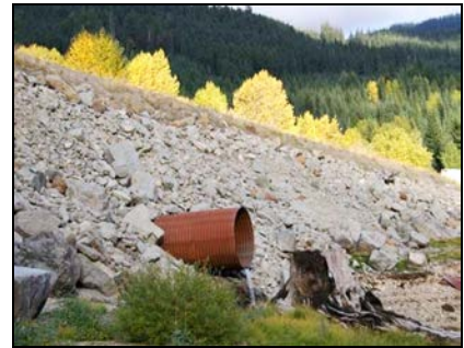
Culverts in the project area can create barriers to fish passage. (Shown: “perched” culvert at Resort Creek)
