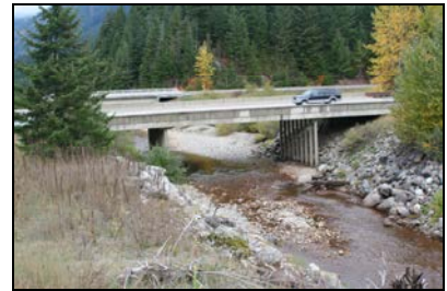
Throughout the project area, bridges and culverts have created artificially confined stream channels. (Shown: Gold Creek)
