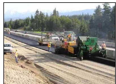
The deteriorated state of the highway requires WSDOT to overlay the pavement with asphalt frequently, causing traffic delay and adding to costs.
