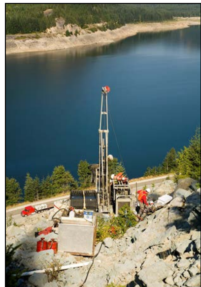
Geotechnical crews evaluate rock for design concerns and potential use in road construction. (Shown: Slide Curve)
