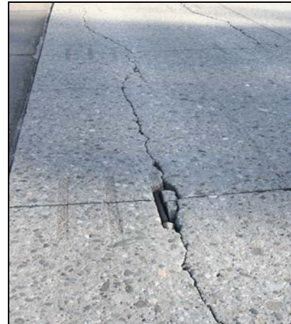
Pavement in the project area has outlived its intended lifespan and is deteriorating rapidly.
