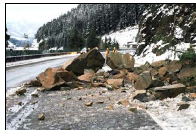
Unstable slopes in the project area regularly lead to rock fall.
