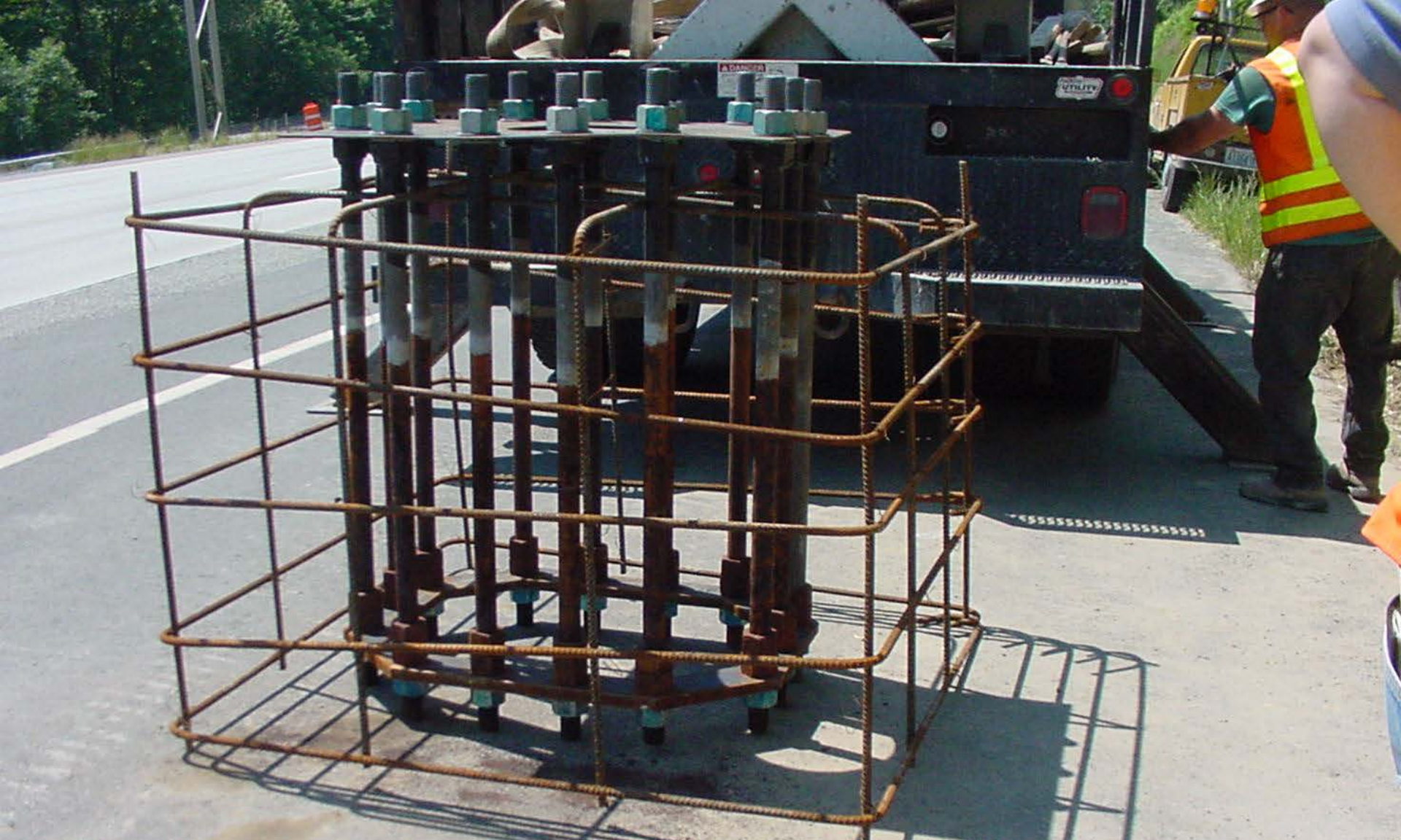
High Mast Bolts and Top Cage
