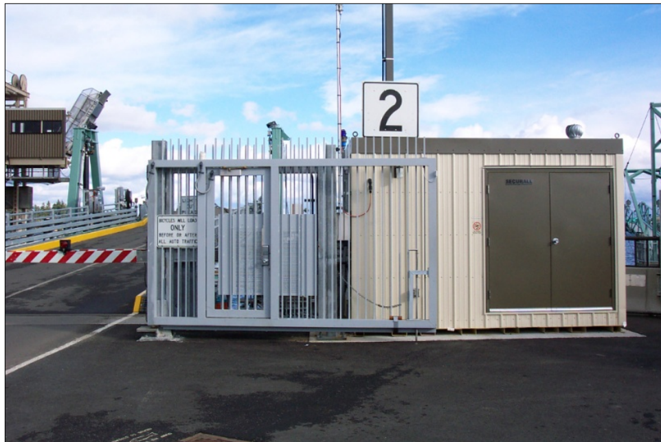
Bainbridge Island Ferry Terminal VTS HPU Enclosure Exhibit 440-17
