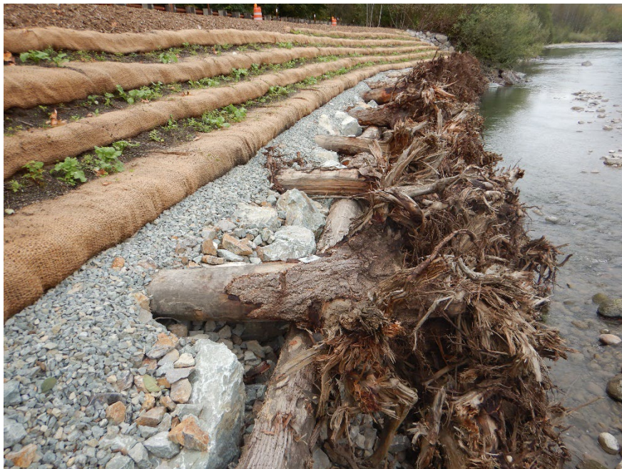
Figure 10A-6 Crib Wall with Soil Lifts (No Piles), Sauk River, Skagit County
