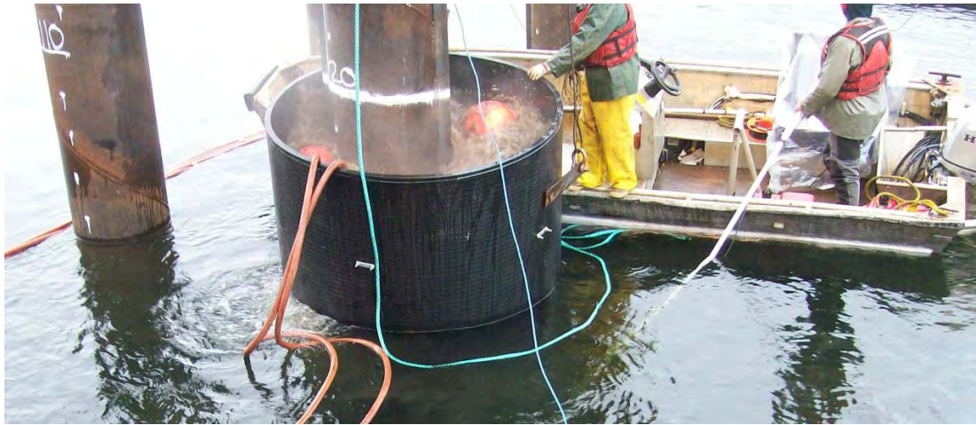
Figure 11: Photograph of bubble action in the isolation casing
