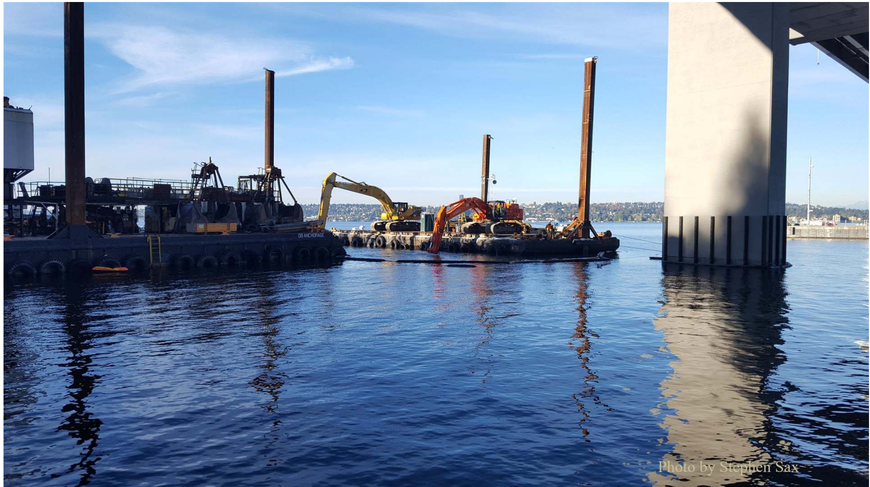
Figure 2: The Relative Locations of the Hoe Rams during Monitoring of the piers
