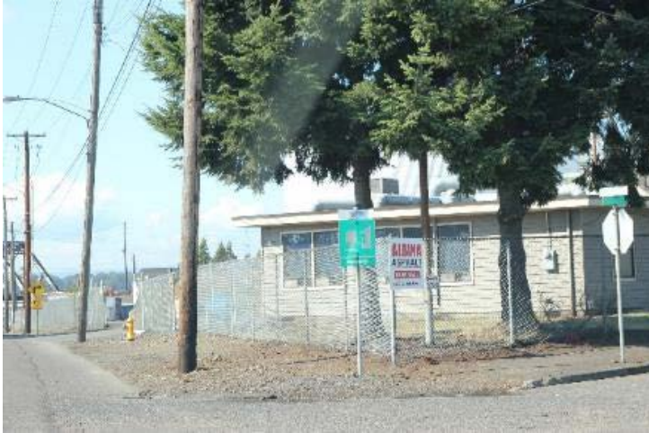
Corner of Hill and 8th Street. Sidewalk in poor condition with no connectivity.
