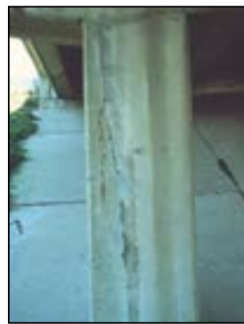
Figure 139. Crack in Pier 3 column. Location 3.
