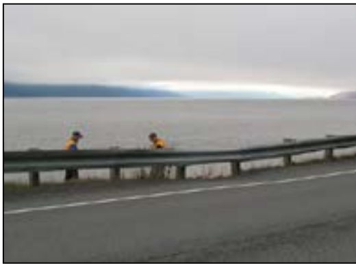
Figure 142. Roadway settlement over pipe culvert. Location 2. (Source: Alaska DOT)
