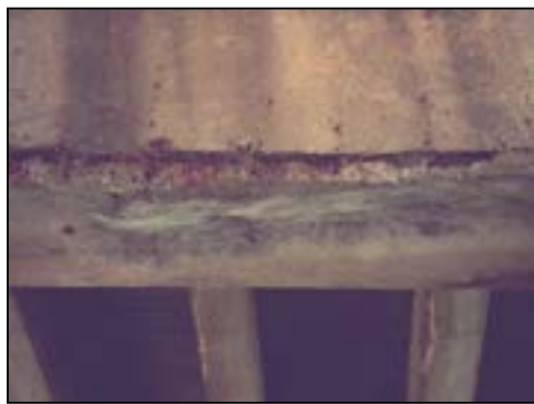
Figure 138. Spall in Pier 2 cap beam. Location 1.
