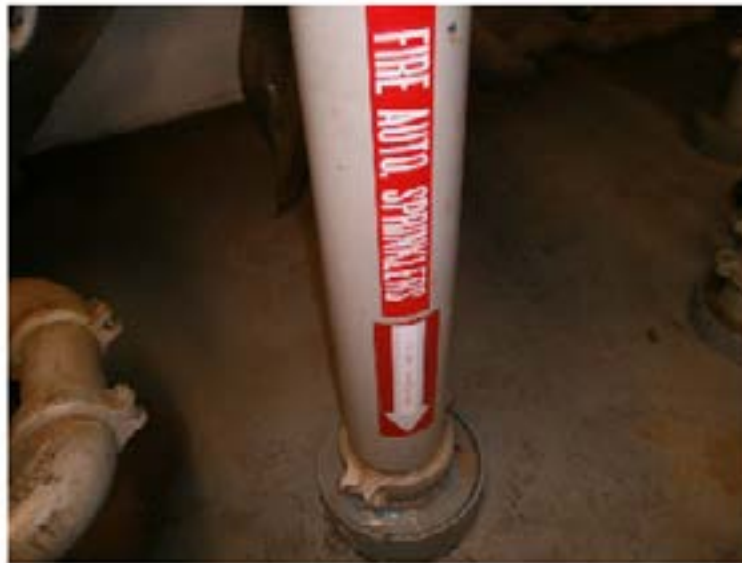
Photo 2 Standpipe Labels – non-compliant with ANSI/ASME A13.1
