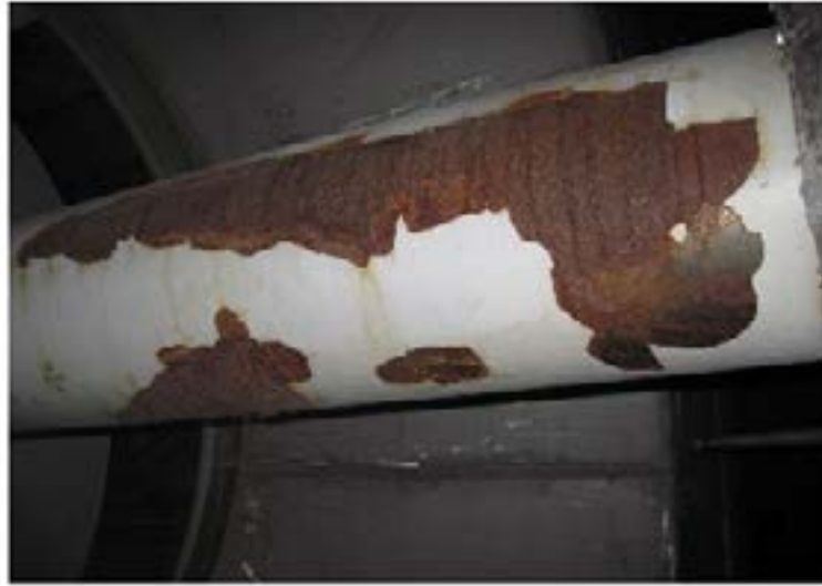
Photo 1 Exhaust Fan Shaft – paint peeling and blistering (typical)
