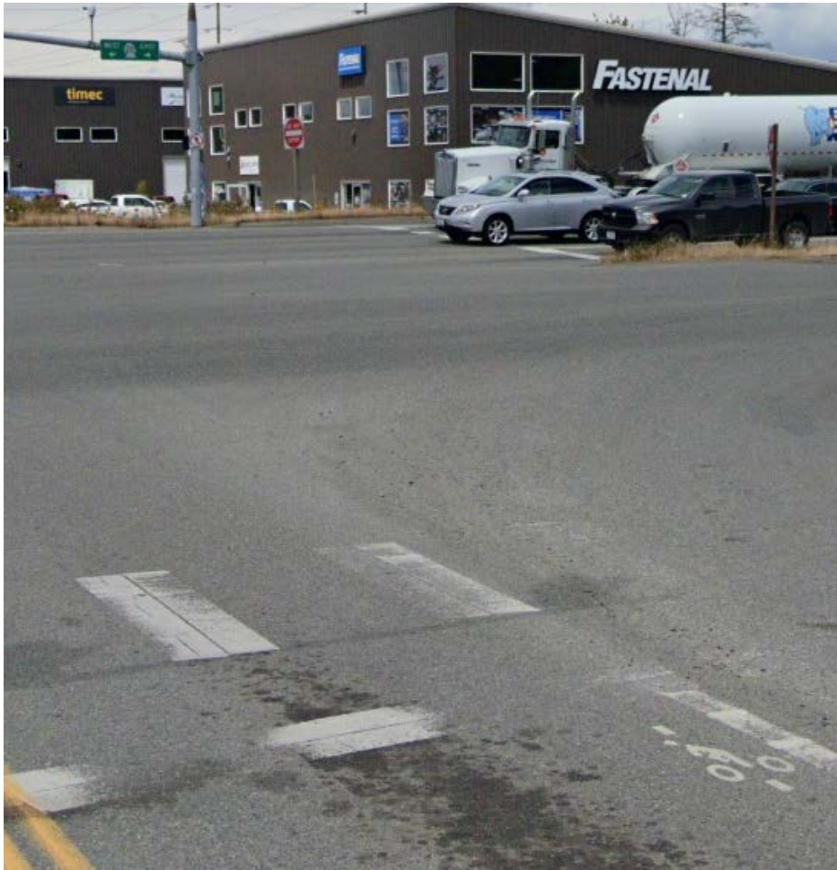
Figure 3-26: Traffic signal detection for bicyclists. The bicycle rider stencil helps riders position their bikes in the intersection so they are detected by the traffic signal and given an opportunity to cross. This detector is located at Reservation Road and SR 20 in Skagit County.
