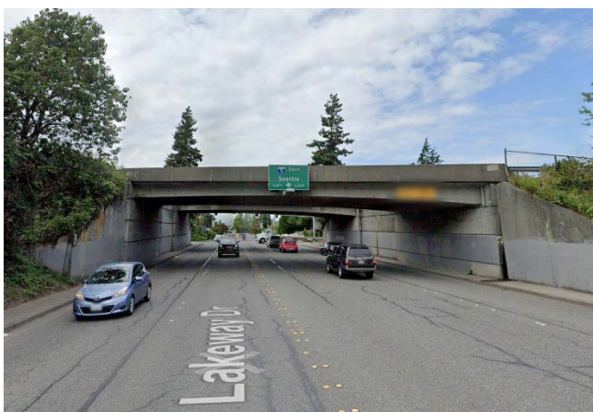
Figure F-23: Bridge gap in Bellingham not identified through network analysis approach to finding network gaps. Bridge 5/809W on I-5 passes over Lakeway Drive. I-5 at this location is prohibited to pedestrians and bicyclists, so it was not identified as an active travel gap. Bridges associated with active travel gaps were identified, but the presence of such gaps was only evaluated on the state highway system. This underpass connects the Western Washington University district to residential and commercial areas of Bellingham. It has sidewalks but no bike facilities. With five lanes and freeway ramps the location presents a local system barrier for pedestrians and bicyclists. The city has expressed interest in improving active transportation connections here.
